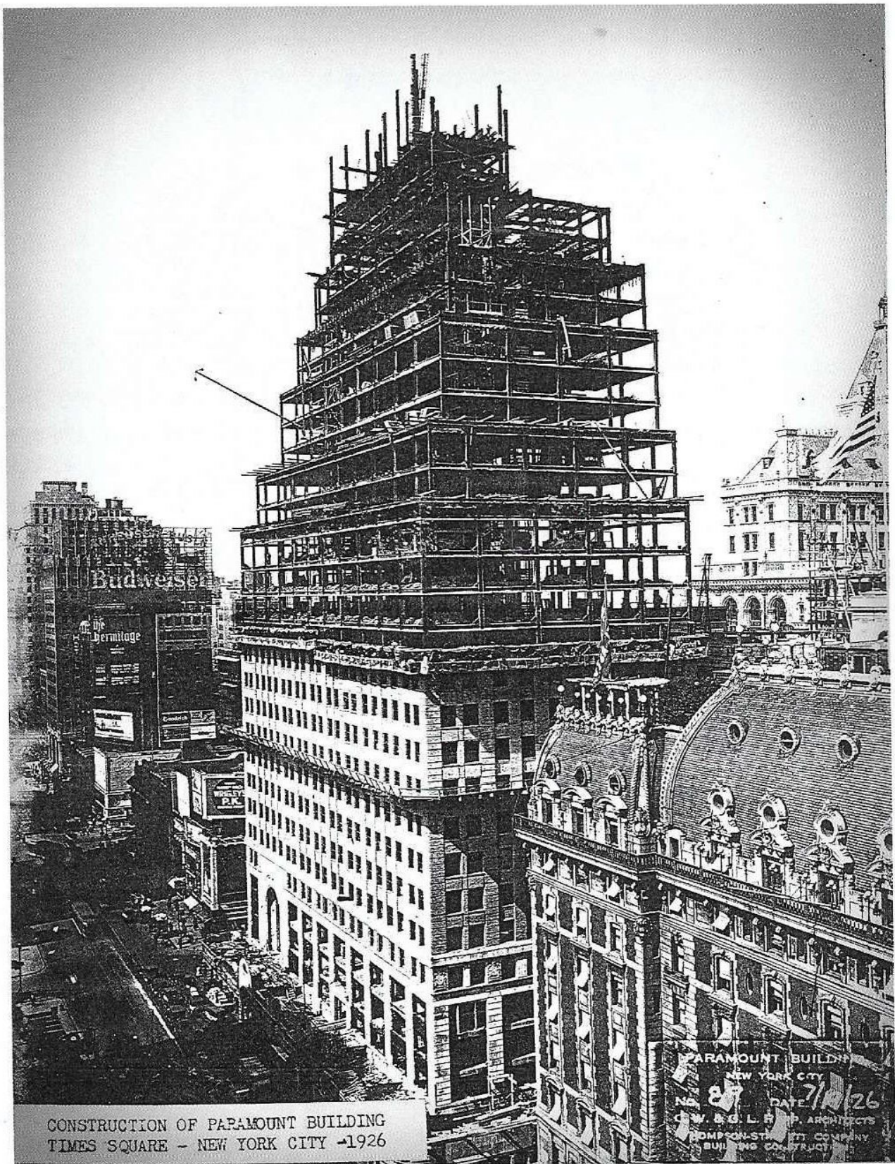
Paramount Building going up in 1926 at Times Square, New York City. To the right is the Astor Hotel where Rapp & Rapp rented rooms for offices during construction. (Rapp Collection)
